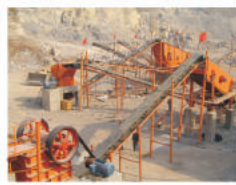
500 TPH CRUSHER PLANT
