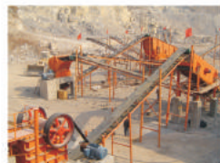
500 TPH CRUSHER PLANT
